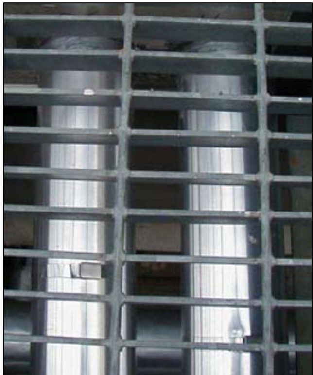
Fig 4. Heat tracing of lube-oil lines minimizes the possibility of thermal cycling
